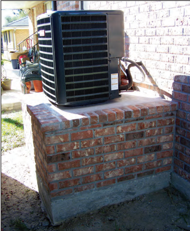
Figure 3-1. Air conditioning compressor elevated on a pedestal.
